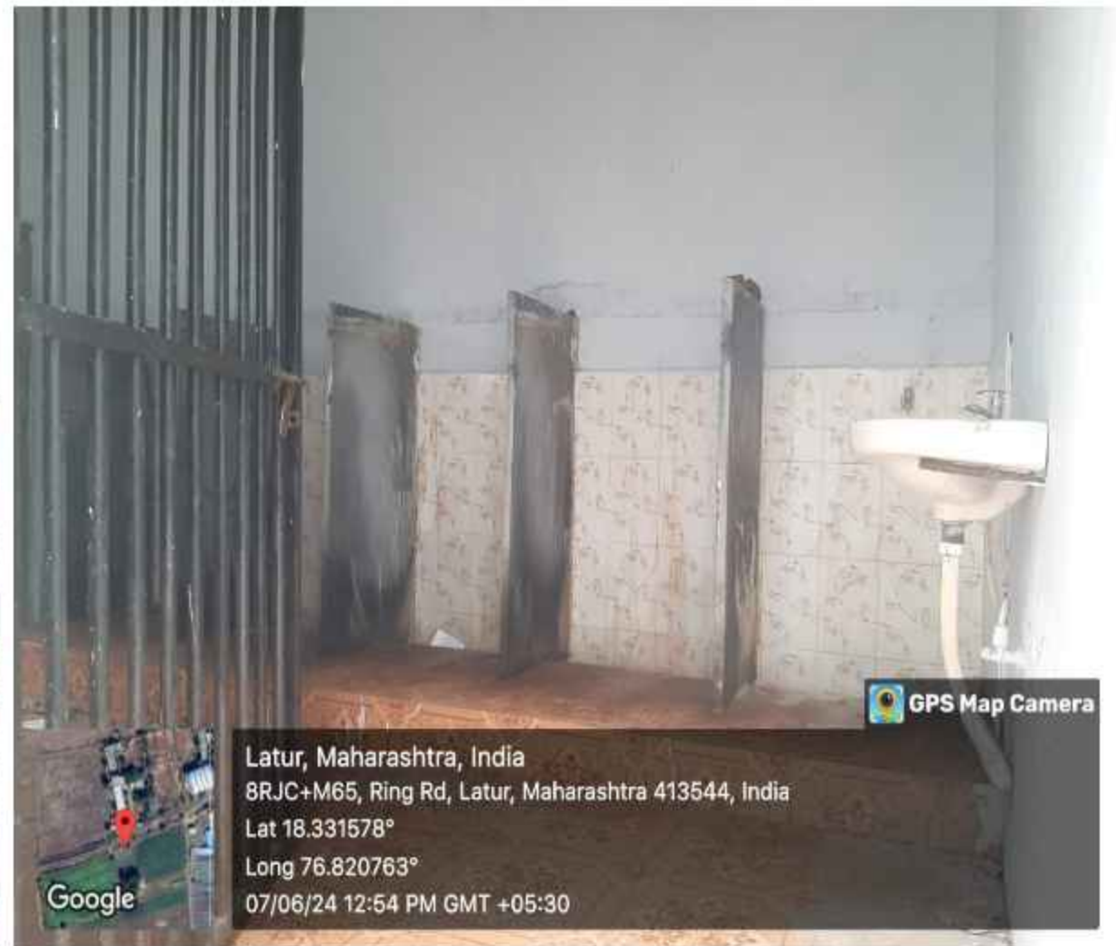
Gents washroom Facility
